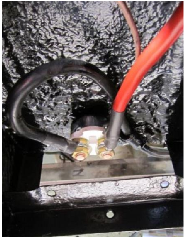
View looking down through the battery cover – the black cable runs from the new switch under the car and forward to the starter motor. The thinner brown wire runs into the car and forward along the tunnel to provide a permanent (unswitched) supply to the radio.
